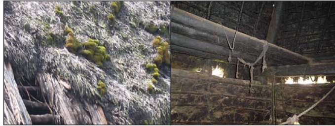
Pic. 24: roof damage
