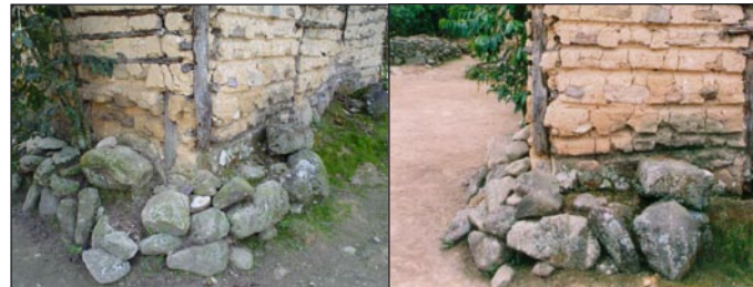
Pic. 14-15 Make-shift wall support of stones
